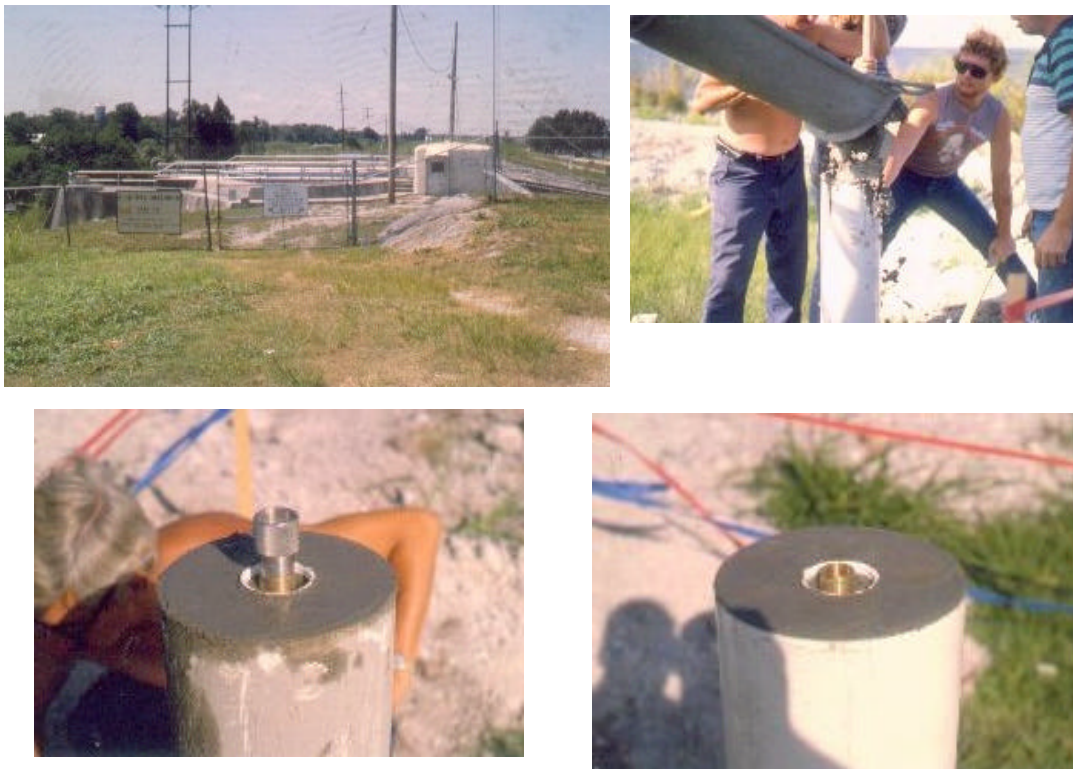
Figure 2-7. Reference point monumentation. Concrete pier construction vicinity of a hurricane gate structure. Forced centering plug set into concrete pier. (Jacksonville District)
